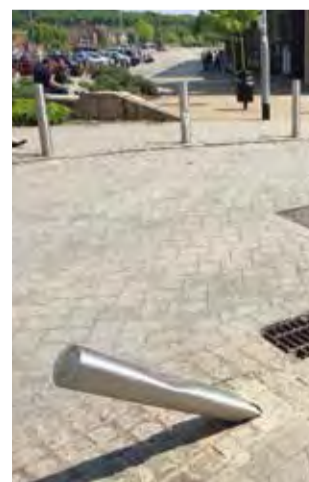
Need to provide robust / low maintenance street furniture
